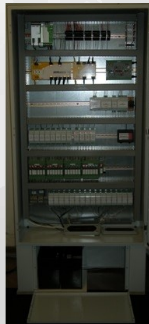
ELC - Electronic Level Crossing
